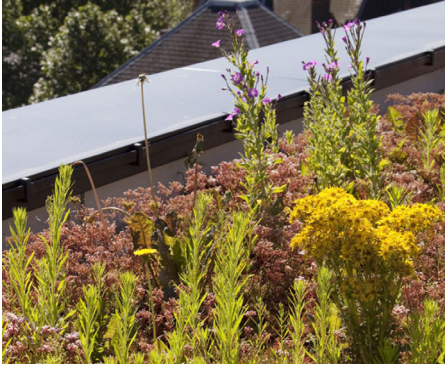
Above: Extensive Wildflower Green Roof finishes provide biodiversity accreditation to a flat roof specification.
